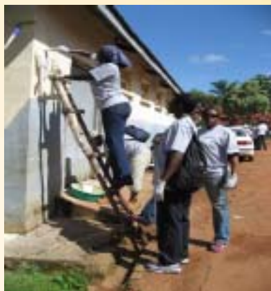
UNVs Mabel Turyagenda and Moses Opio (R, 2nd right) await their turn as Stella Suffer (on ladder) applies a coat of paint on the hospital building
